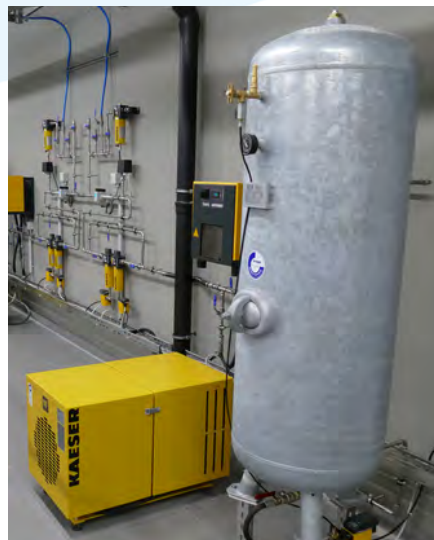
Compressor or control air system
