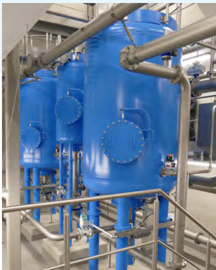
Oxidator and iron removal filters
