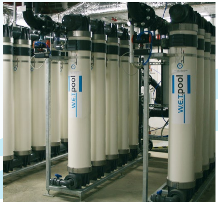
Circular treatment with ultrafiltration
